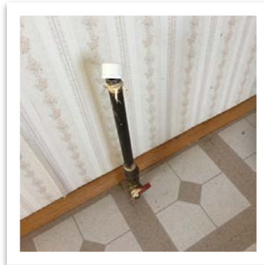
Incorrect type of gas line cap.
