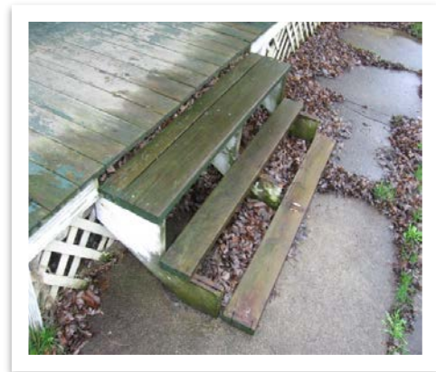
Damaged/missing treads and risers.
