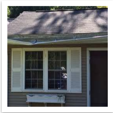
Section of gutter needs repair.
