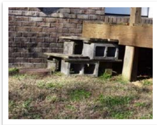
Unacceptable use of materials.
