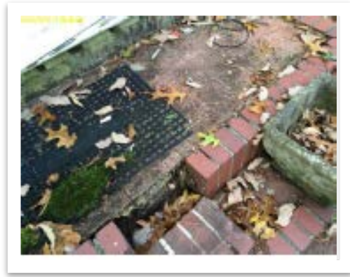
Bricks used for a riser are missing creating a trip hazard.
