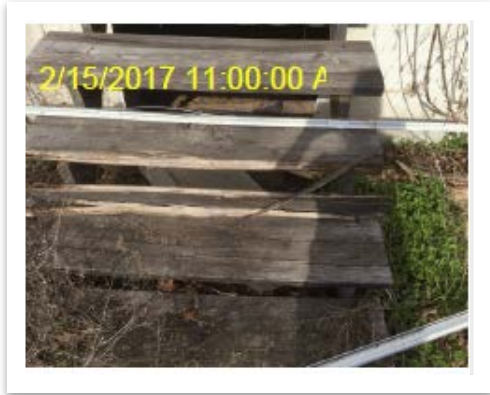
Damaged treads and risers.
